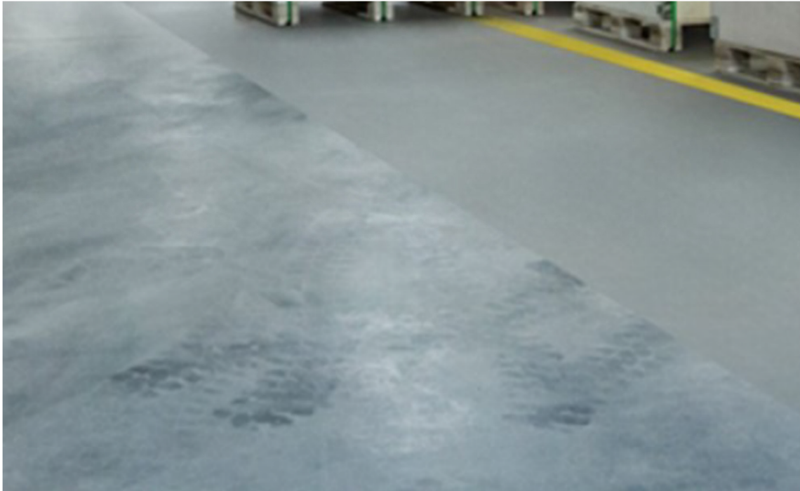
Damaged floor coatings can often be refurbished with minimal effort. Photo: StoCretec
