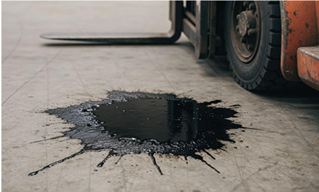
Oil-contaminated floor areas are a common problem in industrial plants. Photo: KI
