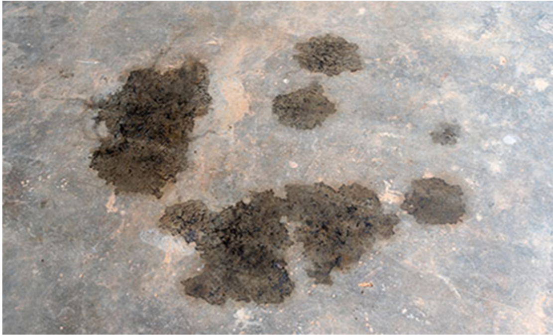
Floor of an industrial hall contaminated with oil. Photo: Adobe Stock
