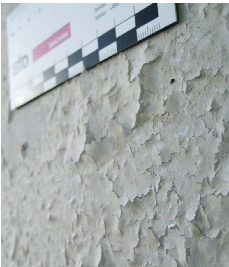
Flaking carrier material, bentonite, following application of the StoCryl HG 200 deep-acting hydrophobic agent
