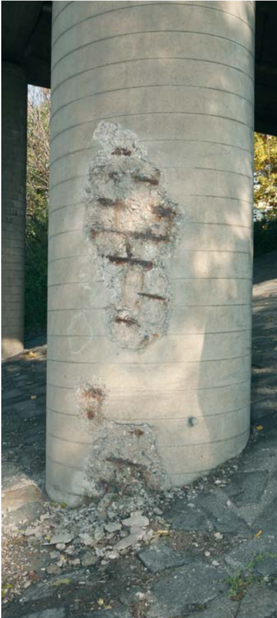
Bridge pier shows damage caused by chloride-induced reinforcement corrosion. Photo: Wacker Chemie AG
